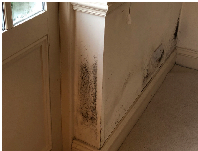
Mould and condensation problems around window reveals and corners
